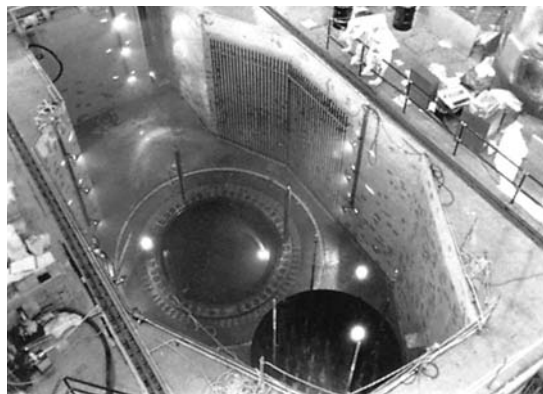
Figure 31 Looking down into the water-filled refueling cavity of the reactor. (Courtesy of Connecticut Yankee Atomic Power Company; photo by Georges Betancourt)
