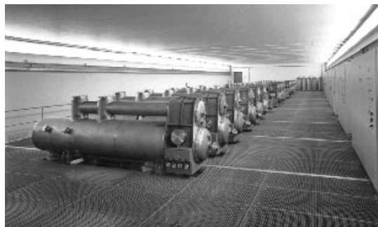
Figure 7 Group of 15 totally enclosed SF 6 circuit breakers installed in an underground substation of a large city. Rated current: 1600 A; rupturing current: 34 kA; normal operating pressure: 265 kPa (38 psi); pressure during arc extinction: 1250 kPa (180 psi). These SF 6 circuit breakers take up only 1/16 of the volume of conventional circuit breakers having the same interrupting capacity. (Courtesy of ABB)
