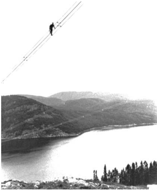
Figure 7a Four bundled conductors make up this phase of a 3-phase, 735 kV line. (Courtesy of Hydro-Québec)
