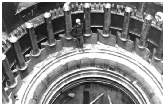
Figure 12 Inside the spiral case, a set of adjustable wicket gates control the amount of water flowing into the turbine. (Courtesy of Marine Industrie)
