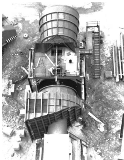
Figure 19 This forced-draft fan provides 455 \text{ m}^3/\text{s} of air at a pressure difference of 5.8 kPa for a thermal power station. It is driven by a 3-phase induction motor rated 12 000 hp (8955 kW), 60 Hz, 890 r/min. (Courtesy of Novenco Inc.)
