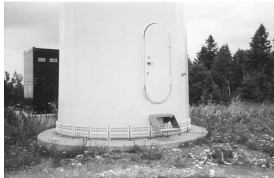
Figure 38c The base of the steel tower has a diameter of 4.5 m. The door gives access to the inside and upwards to the nacelle. The transformer connecting the turbine to the 230 kV grid can be seen in the background. The connection to the grid is made by means of an underground cable.
