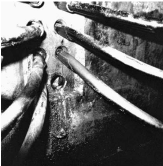
Figure 27 MV underground feeders in concrete duct.
