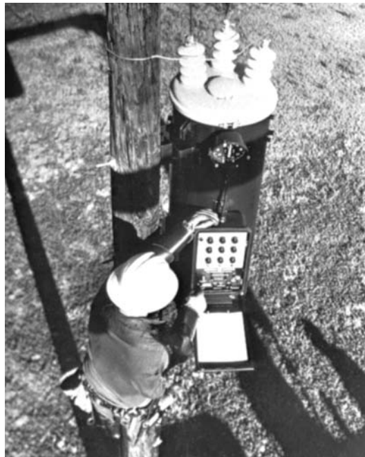
Figure 29 Automatic tap-changing autotransformer maintains steady voltages on long rural lines. (Courtesy of General Electric)
