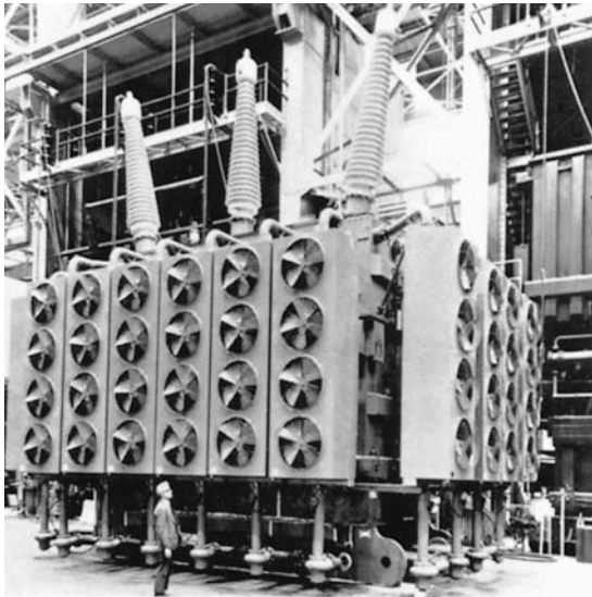
Figure 18 Three-phase, type FOA, transformer rated 1300 MVA, 24.5 kV/345 kV, 60 Hz, 65°C temperature rise, impedance 11.5%. This step-up transformer, installed at a nuclear power generating station, is one of the largest units ever built. The forced-oil circulating pumps can be seen just below the cooling fans. (Courtesy of Westinghouse)
