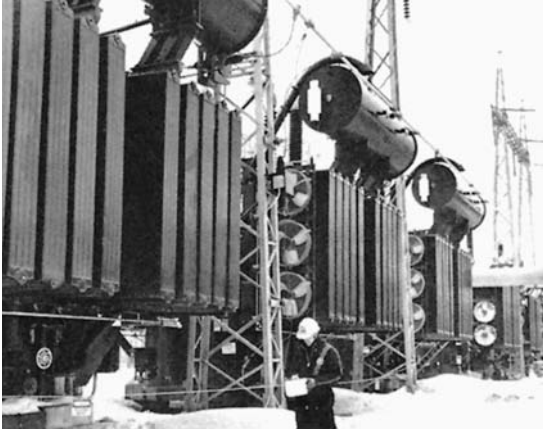
Figure 14 Three-phase converter transformer bank rated 230 kV/ 127 kV/17 kV composed of 3 single-phase transform- ers each rated 323 MVA. (Courtesy of Manitoba Hydro)
