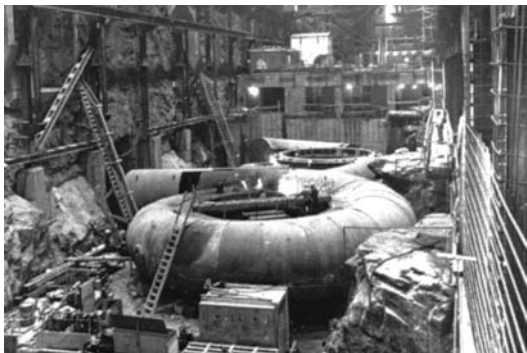
Figure 11 Spiral case feeds water around the circumference of a 483 MW turbine. (Courtesy of Marine Industrie)
