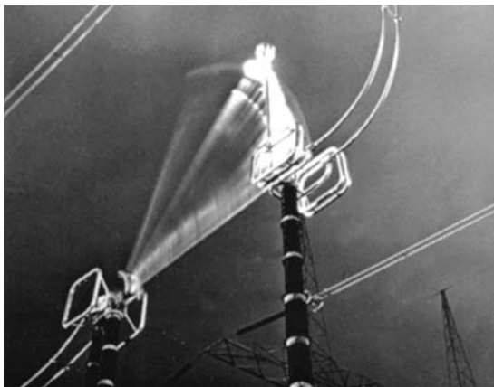
Figure 11 The arc produced between the horns of a disconnecting switch as it cuts the exciting current of a HV transformer provides the light to take this night picture. (Courtesy of Hydro-Québec)
