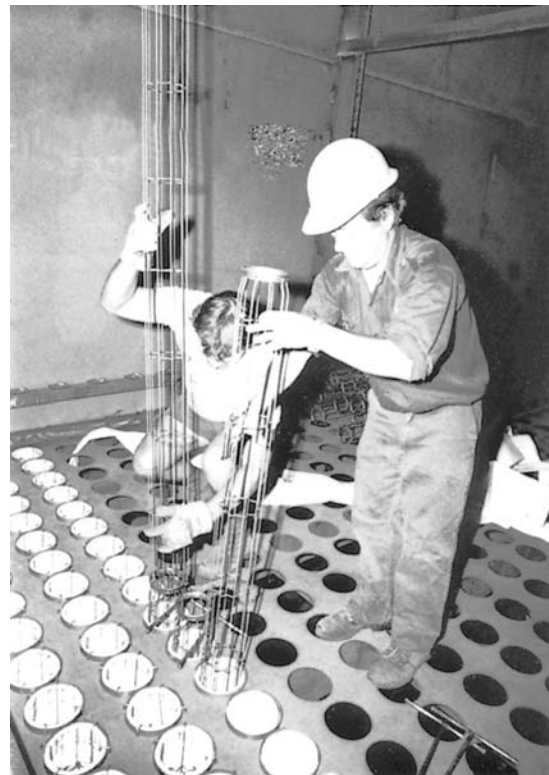
Figure 27 Installation of the fabric filter bags. Each bag is 15 m long and 16 cm in diameter. (Courtesy of Electricity Commission of New South Wales)
