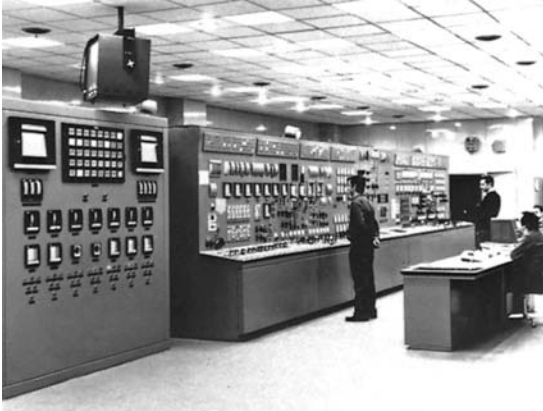
Figure 23 Control room of the 540 MW generator set. (Courtesy of General Electric)
