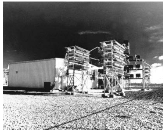
Figure 39 Static var compensator for HV line. (Courtesy of General Electric)
