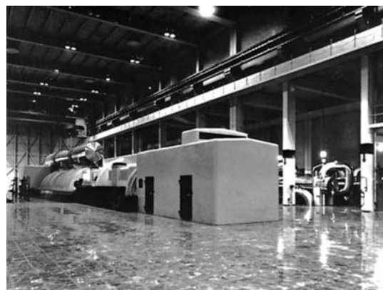
Figure 22 This 540 MW steam-turbine generator set runs at 3600 r/min, generating a frequency of 60 Hz. The low-pressure turbine and alternator are in the background. (Courtesy of General Electric)
